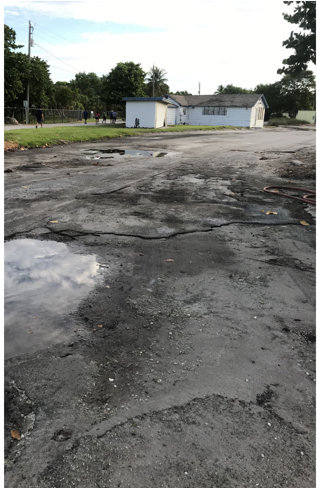
Adjacent road to Cabana's parking in very poor condition
