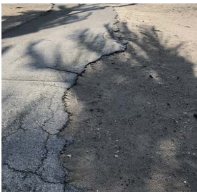
Cracked road edge
