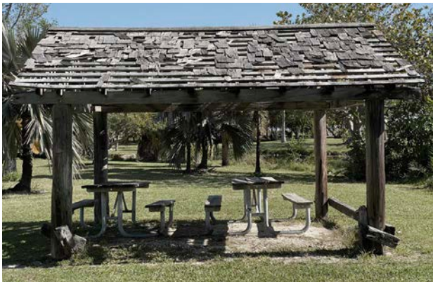
Crumbling Picnic Shelter
