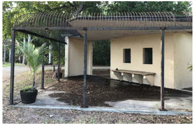
Poorly maintained structures
