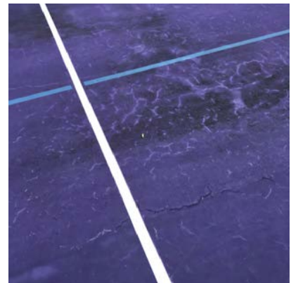
Cracked tennis courts
