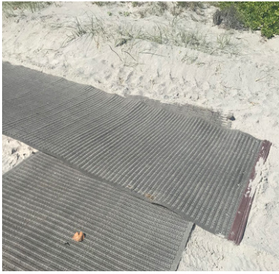
The only ADA access to beach in poor condition
