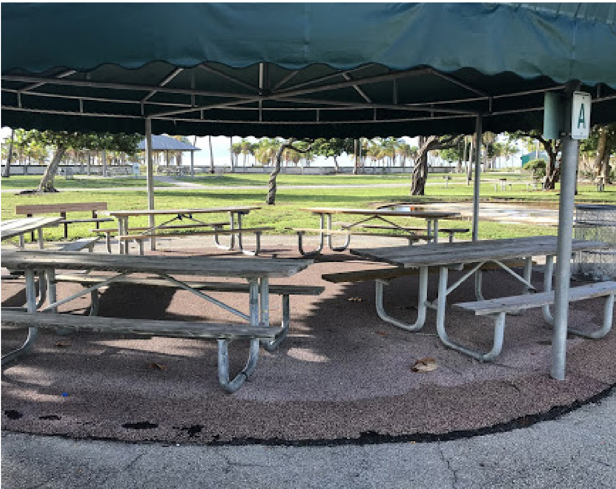
Picnic Carousel in Amusement Center is in poor condition
