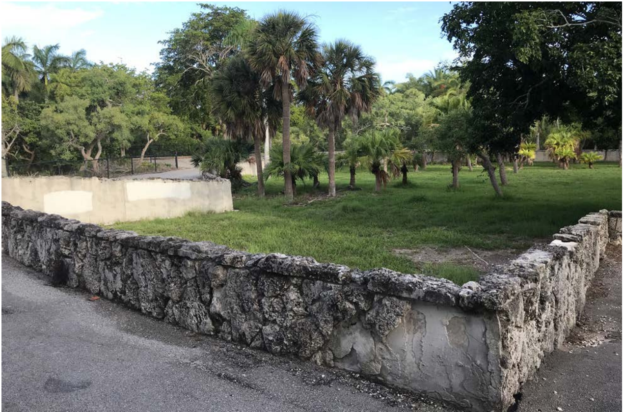
Crumbling walls in the Overlook
