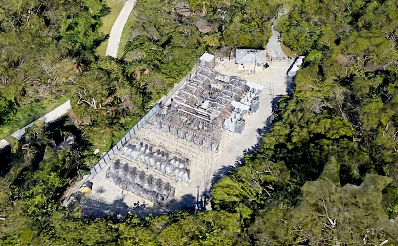
Substation is located near Calusa Park on the west side of Crandon Boulevard.
