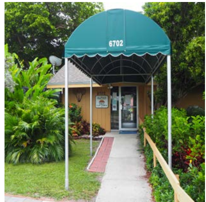
Arraya Tennis club entrance and amenities are in poor condition
