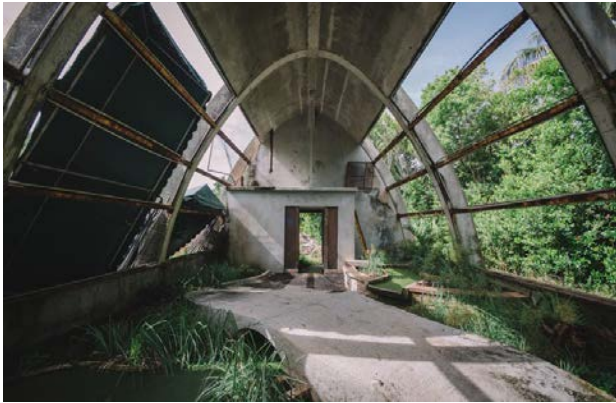
Abandoned structures that is inaccessible to the public
