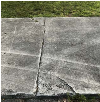
Cracked concrete sidewalks
