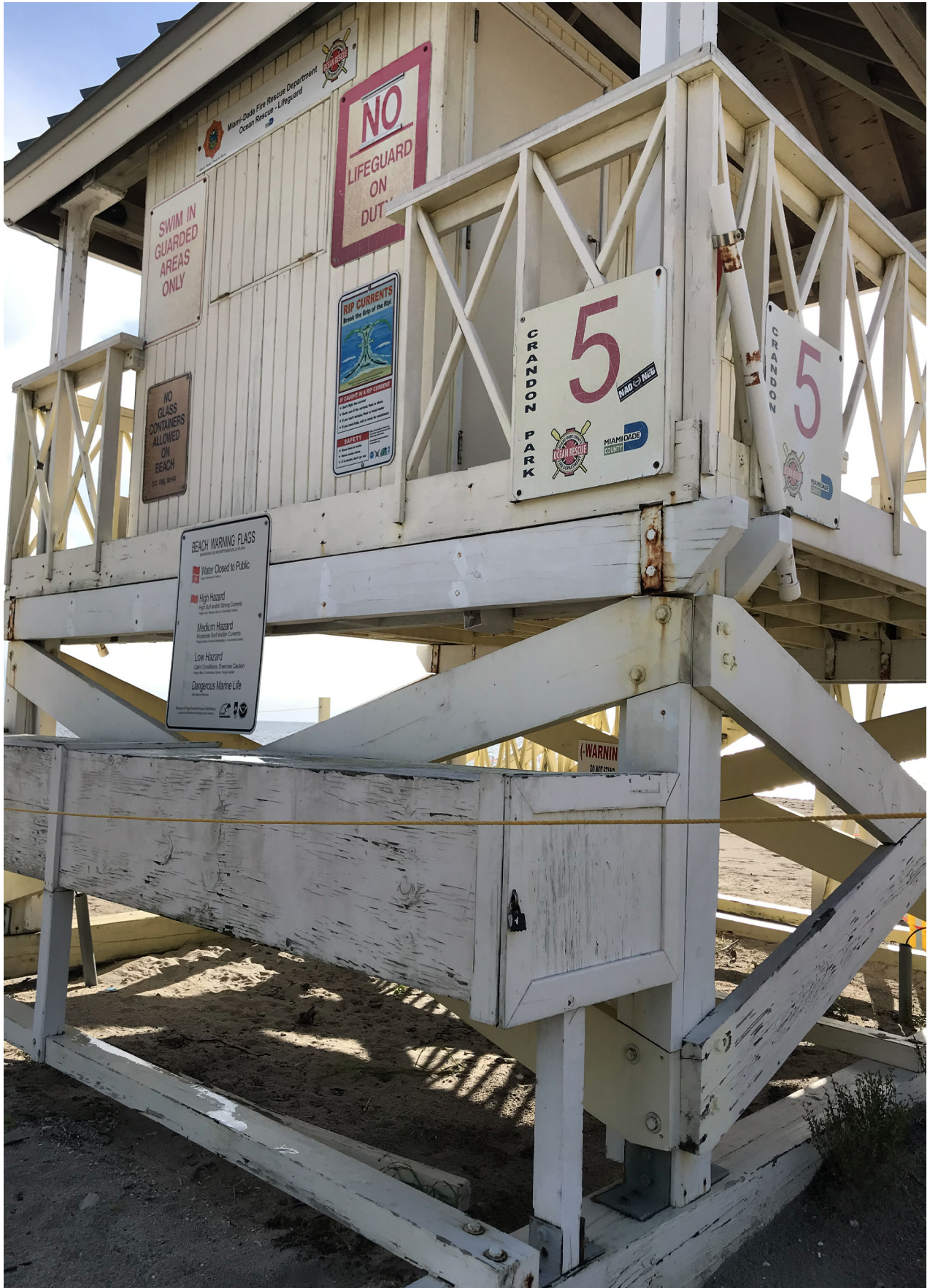
Lifeguard stations are in need of refurbishment
