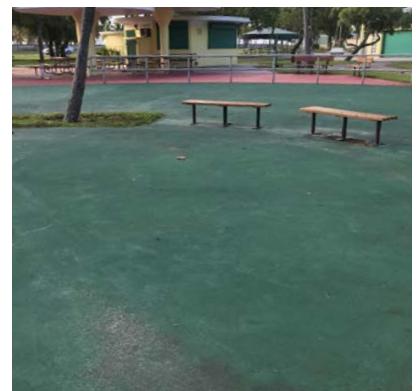
Playgrounds in poor condition
