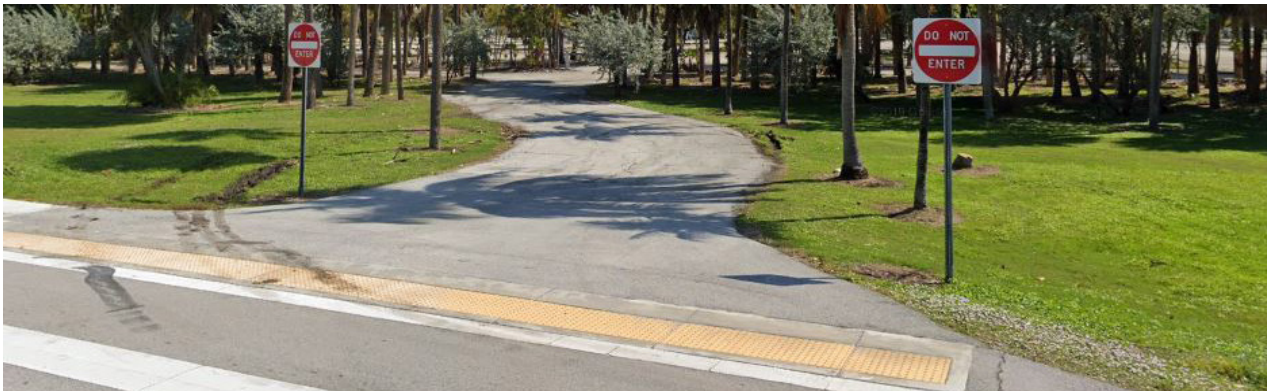
Asphalt pedestrian path is confusing for drivers since path width and materialisation (asphalt) are the same as for vehicles.
