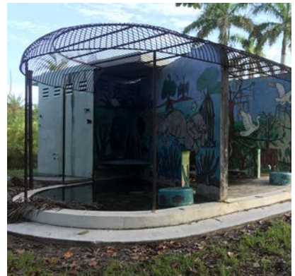
Abandoned zoo structure
