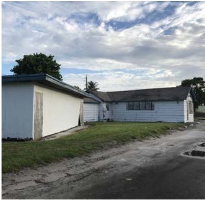
Unknown structures by Cabana area in poor condition
