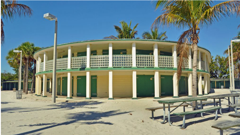
Beach Cabanas are in fair condition and out-dated
