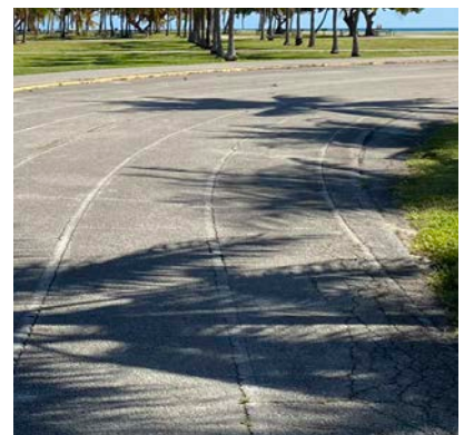
Abandoned track at Central Allée
