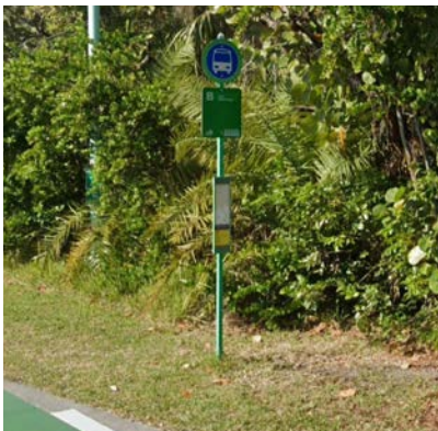
Bus Stop #2 - Sign only, no connection to a sidewalk
