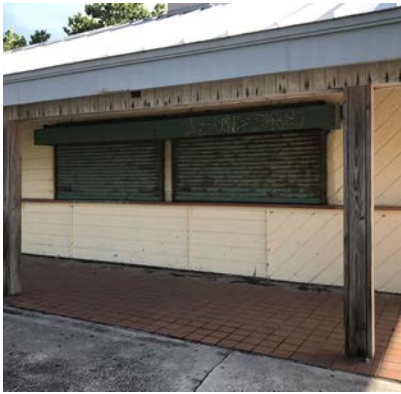
Beach concessions in poor condition and not in use
