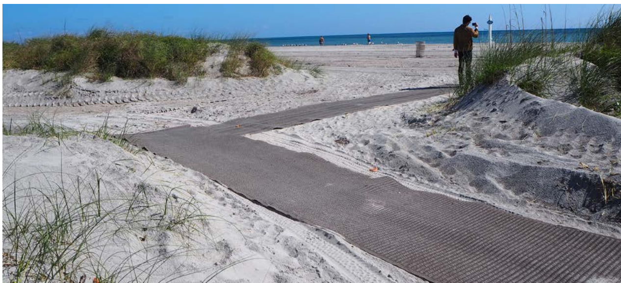
The only ADA path to the Beach in poor condition
