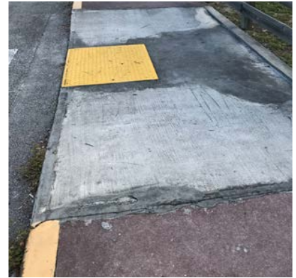
Sidewalk along South Parking Lots in poor condition
