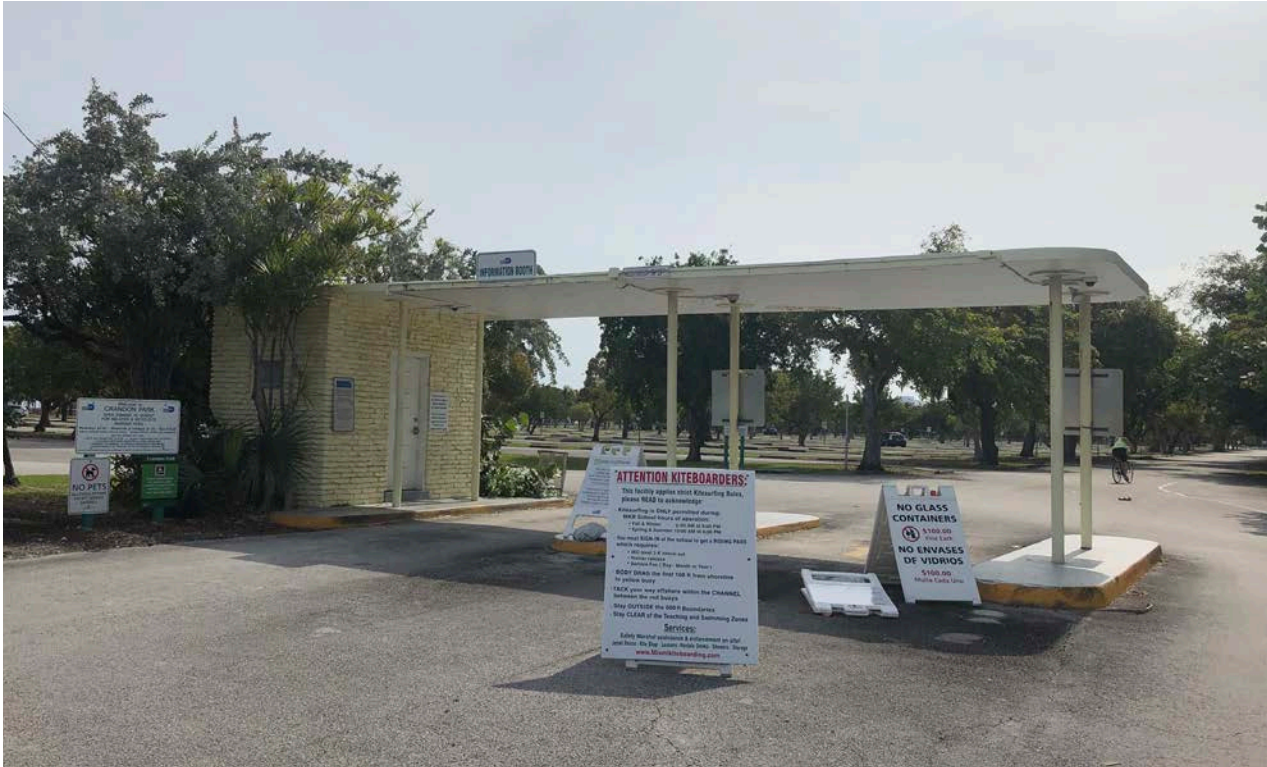
Structure is abandoned and its function is replaced by temporary signage
