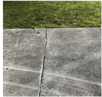
Damaged path in Calusa Park
