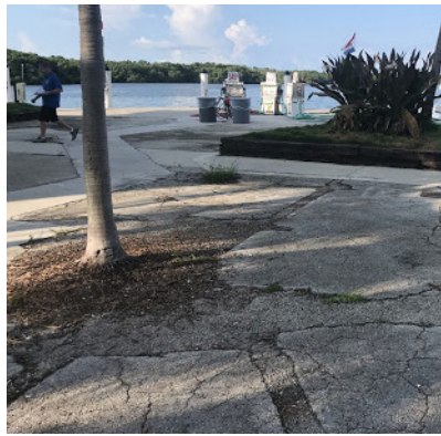
Damaged sidewalk by the Marina office
