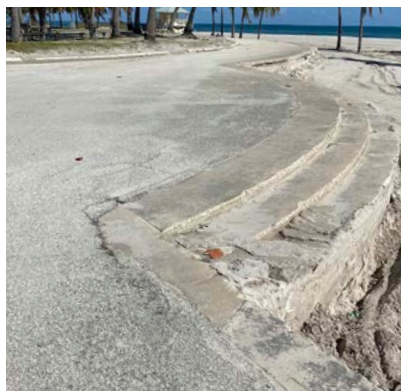
Damaged beach promenade steps
