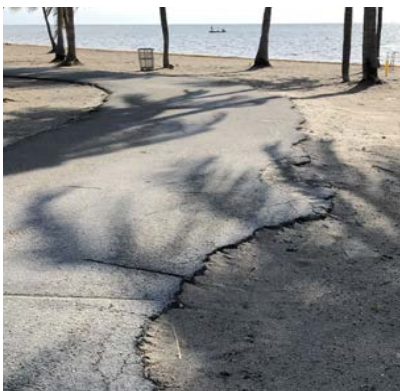
Damaged path at Crandon Beach
