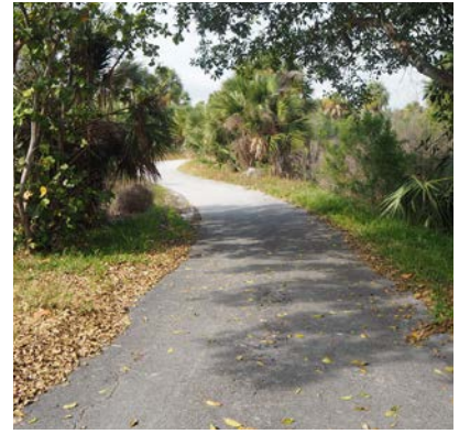
Shared path in Bear Cut Preserve in fair condition and receives some use
