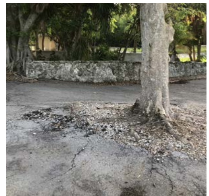
Damaged Path in Crandon Gardens
