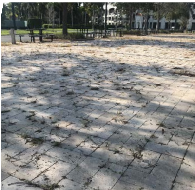
Overgrown paving at Tennis Center, this area is rarely in use
