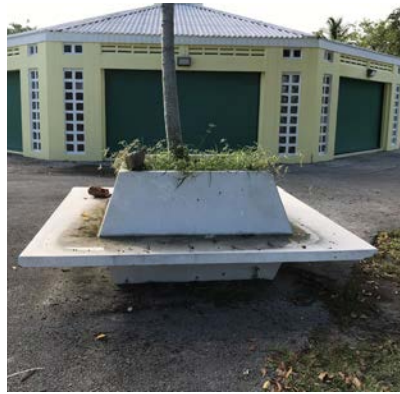
Cabana benches in poor condition
