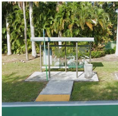
Bus Stop #3 - Shade and bench, no connection to a sidewalk
