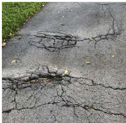
Damaged path in Crandon Park
