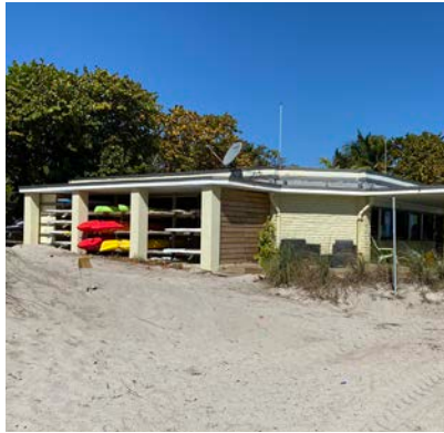
Kayak rental area in poor condition
