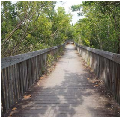
Boardwalk to Fossilized Reef Overlook in fair condition
