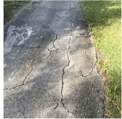
Shared path connecting Key Biscayne village and Crandon Park is in poor condition
