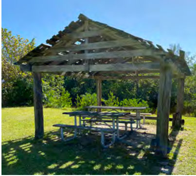
Crumbling picnic pavillion in Crandon Gardens
