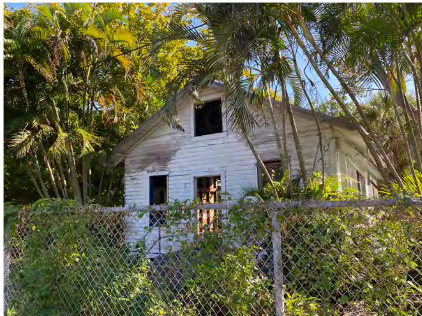
Calusa Playhouse, once an artistic hub in Calusa Park, is now abandoned and inaccessible. Facilities such as these will eventually be torn down.
