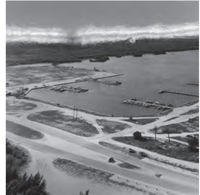
The Marina shown under construction in the 1950s. It was created by dredging the existing wetlands and creating upland for Crandon Boulevard.
